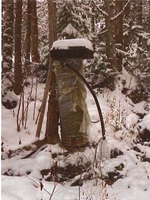
4. Creek intake at PD57252 servicing adjacent property under licence C063512. Water column builds head and accounts for artesian pressure (overflow frozen in photo). View looking east.
