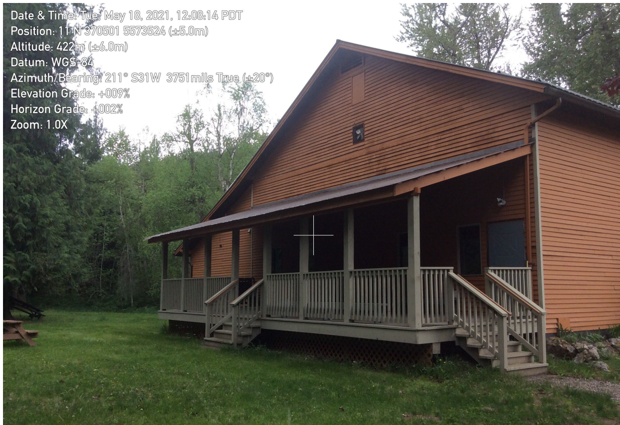
Figure 27: Mabel Lake Community Hall in Tolley Park FireSmart example - could enclose the underside of the deck with fire-resistant material to reduce the risk of embers and sparks collecting underneath and igniting the hall
